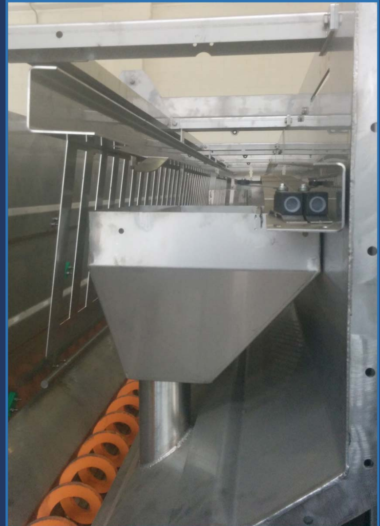
Grease collection system
